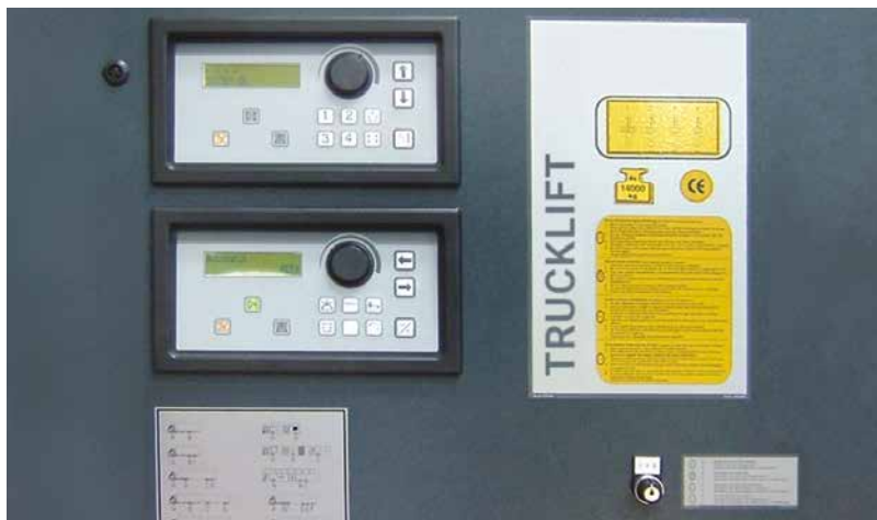
Central control and programming unit with two displays.
